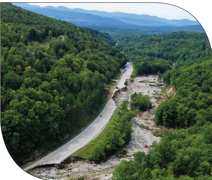
Aerial view of damage along U.S. Route 4 in Mendon, Vermont, as a result of floodwaters from Mendon Brook during Tropical Storm Irene in August 2011. Photograph by the U.S. Geological Survey.
